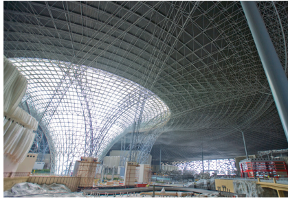
The roof spaceframe and central column will need constant attention. Note the mist, which made cleaning difficult.
